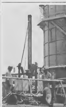
DRILLING FOR oil? Nope, testing coral thickness so foundations can be designed for outboard concrete section additions to increase the efficiency of Combination Units 5 through 8.
